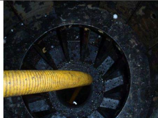
The out nozzle was free cleaned and free of obstruction
