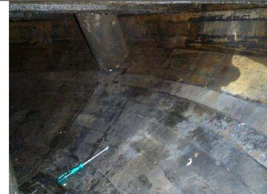
The reactor bottom head lining (clad) was in serviceable condition without visible damages
