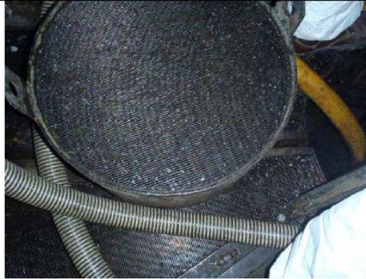
The catalyst support grid center piece was free of mechanical damages.
