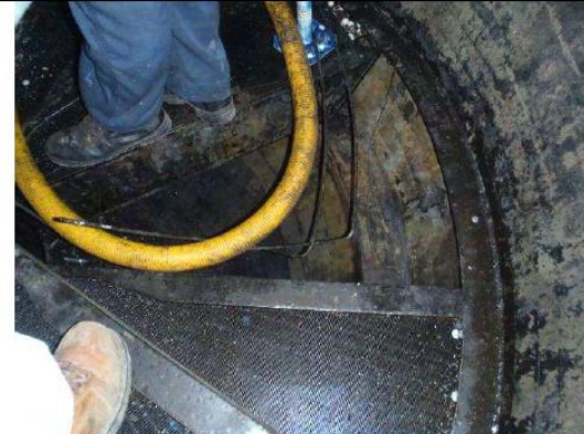
Some pie section of the catalyst support grids were remove to visually inspect and clean the reactor bottom head
