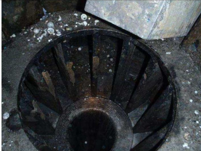
The catalyst support grid support was serviceable
